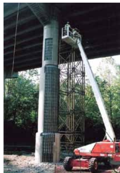
QUIKRETE Shotcrete MS with corrosion inhibitor used in the structural repair of a bridge pier
