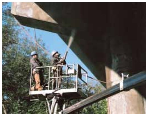
QUIKRETE Shotcrete MS with corrosion inhibitor being applied to a hammer head
