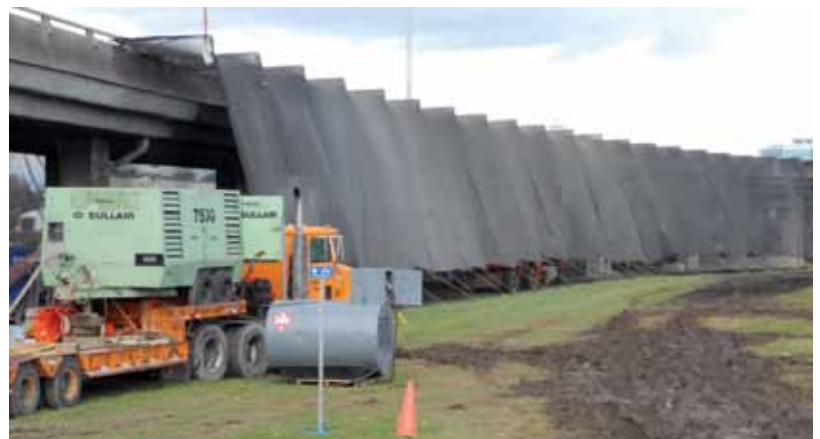
Fig. 5: Netting protected over 280,000 vehicles per day that use the interchange
