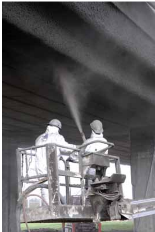
Fig. 7: A repair zone is blasted to clean the reinforcing bar and the substrate
