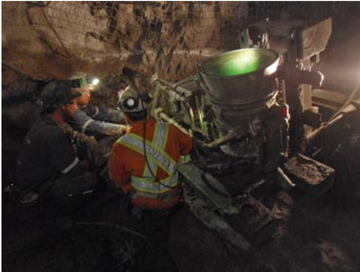
Fig. 4: King representative working with mining personnel to perform maintenance on a dry-mix shotcrete machine
