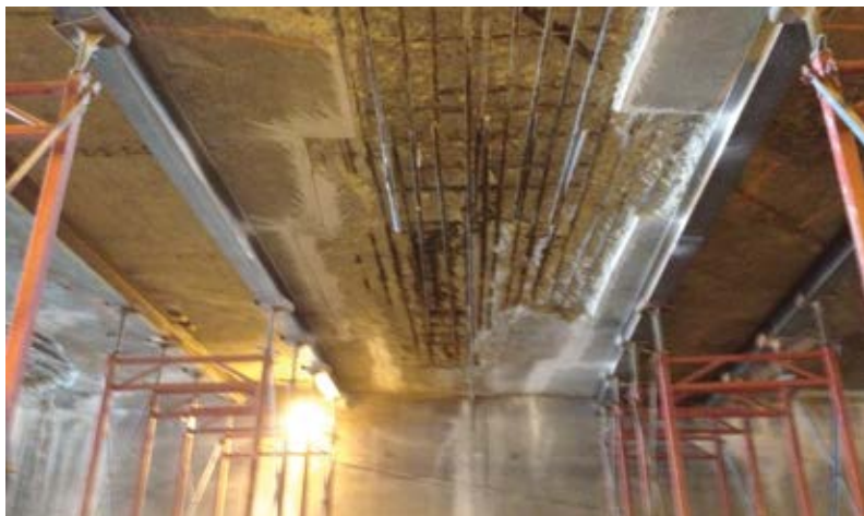
Fig. 1: Shoring towers at 8.5 ft (3 m) apart made for tight access between the exposed deteriorated concrete
