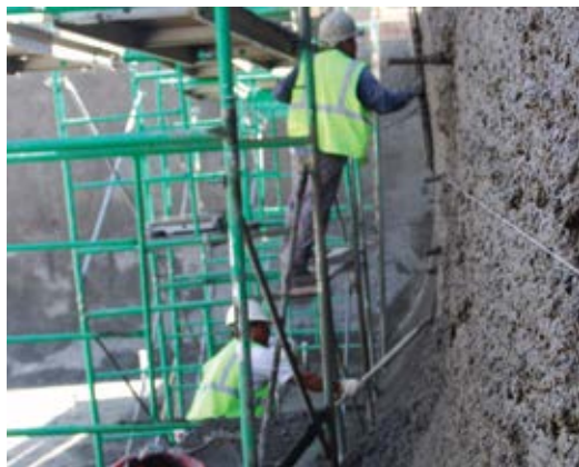
Fig. 3: Pre-job toolbox talks should identify daily risks. Inform workers of the safe operation and use of required tools, such as job-specific scaffolding, before work commences
