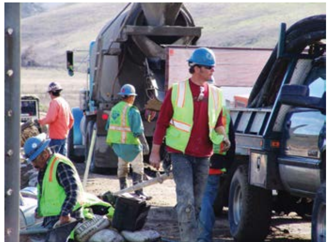
Fig. 2: Job-site meetings or toolbox talks are critical to informing workers of potential safety hazards
