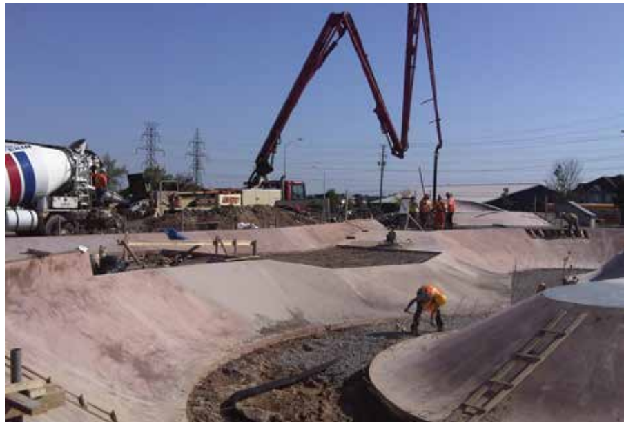
Fig. 4: Ease of equipment access
