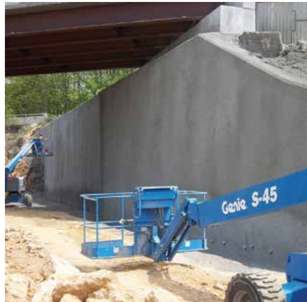
Fig. 5: A float 'finish' was required. The shotcrete depth was greater than 36 in. (914 mm) in some areas
