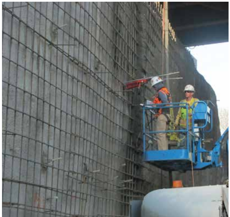
Fig. 3: Manlifts were used to address the wall because scaffolding was not an option so close to the railroad
