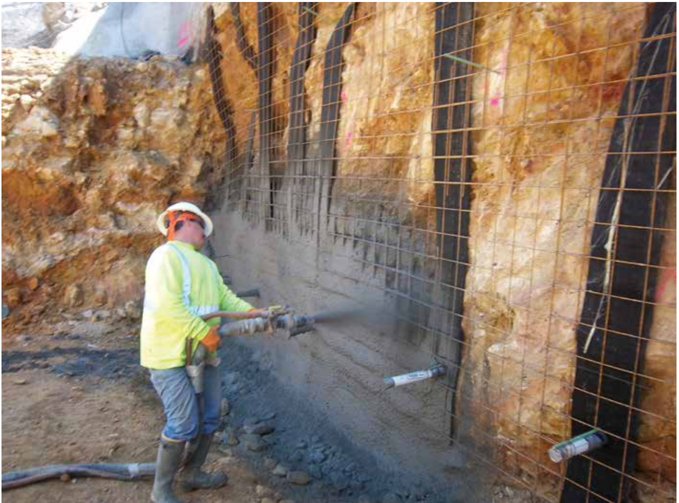
Fig. 2: An initial layer of shotcrete was applied to stabilize the drill bit during the drilling operation
