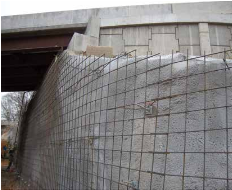
Fig. 4: The finished wall ranged in depth 11 to 24 in. (279 to 610 mm) with two mats of reinforcing steel in some places
