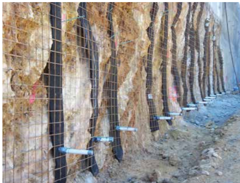
Fig. 1: Drain board and weep pipes were incorporated before applying the shotcrete to allow for drainage
