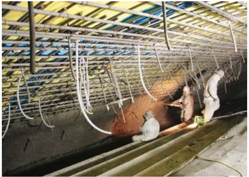
Fig. 2: Overhead arch—lower panel being built up. Note the BA anchors and injection tubes displaying the depth of the concrete section
