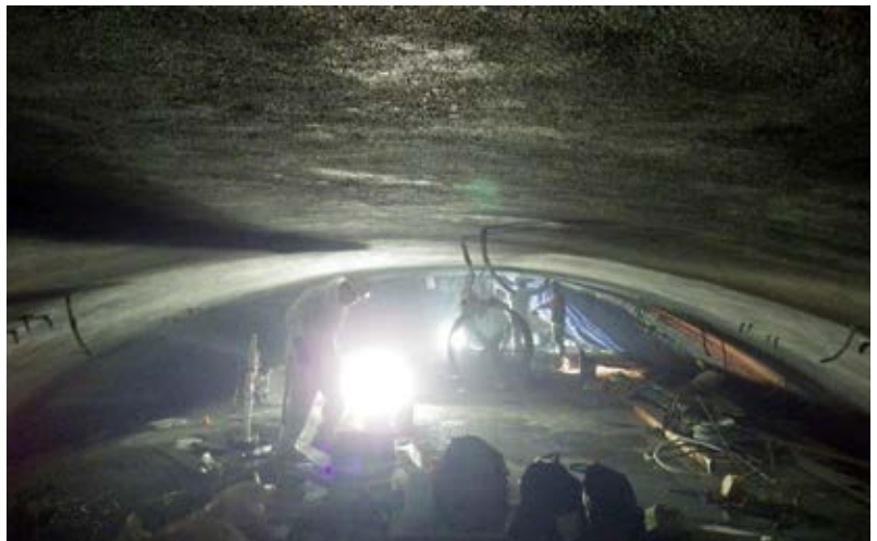
Fig. 3: Working on final panel—heat presented a challenge, requiring ventilation and close attention to curing
