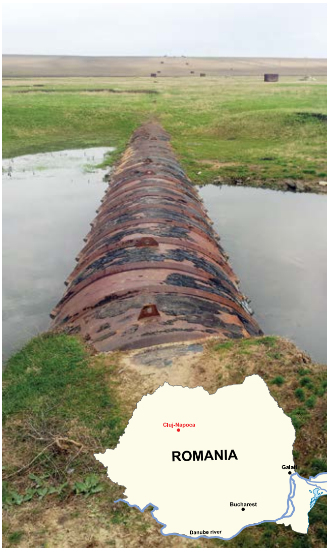
View of one of parallel pipes of Suhurlui Irrigation Pipeline
