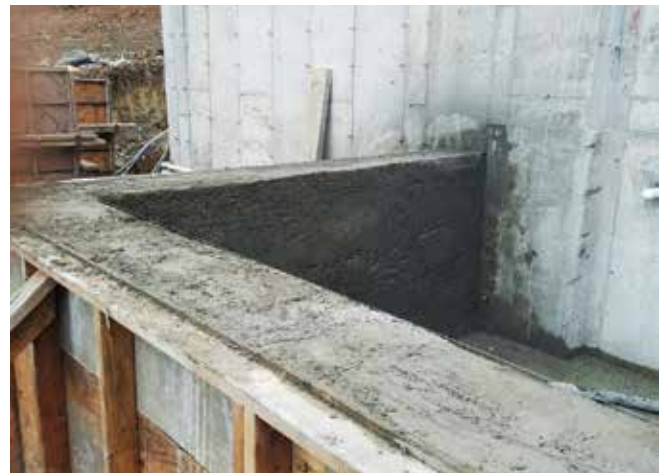
Fig. 4: Wet-mix shotcrete placement against an existing cast-in-place structure created a monolithic, watertight concrete vessel. The marriage of these two placement techniques was completed without bonding agents or expansion joints
