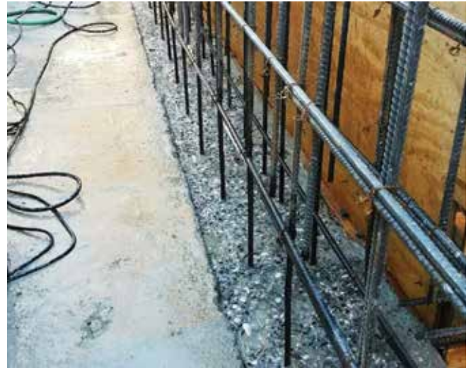
Fig. 3: Reinforcing bars, non-vibrating rigid forming, and a roughened SSD bond plane were installed to connect the cast concrete foundation and the shotcreted portions of the pool structures
