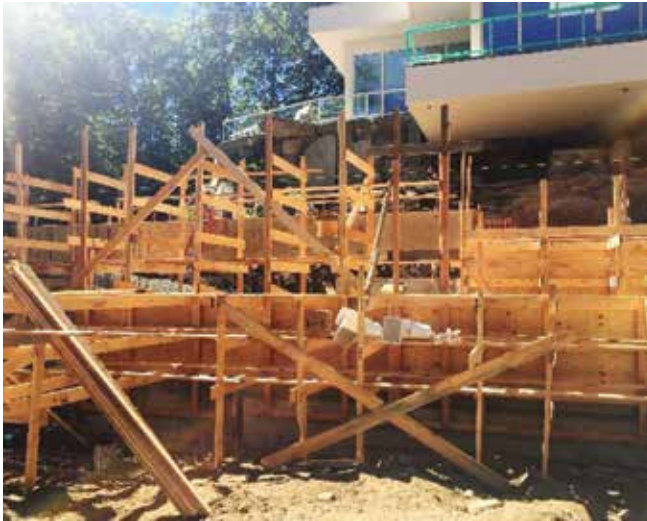
Fig. 2: Although intricate forming was required for this out-of-ground pool construction, the use of sustainable shotcrete resulted in a material savings of 50% due to needing only one-sided forming
