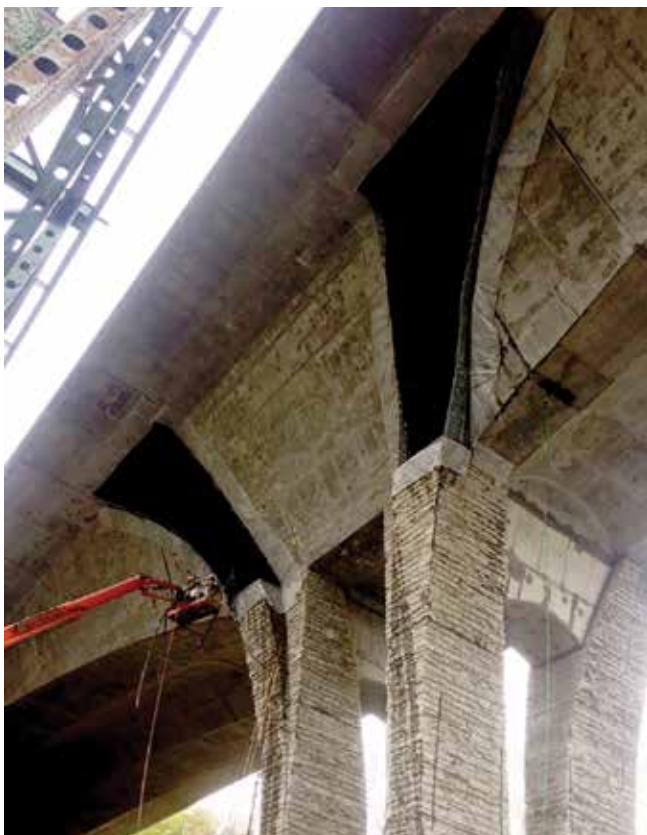
Fig. 1: Two fins at the northern pier prior to being shot. Reinforcing bar and stayform
