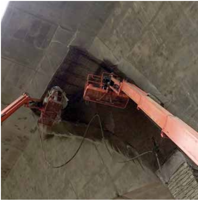
Fig. 5: First day shooting a fin, bringing shotcrete just past the reinforcing bar
