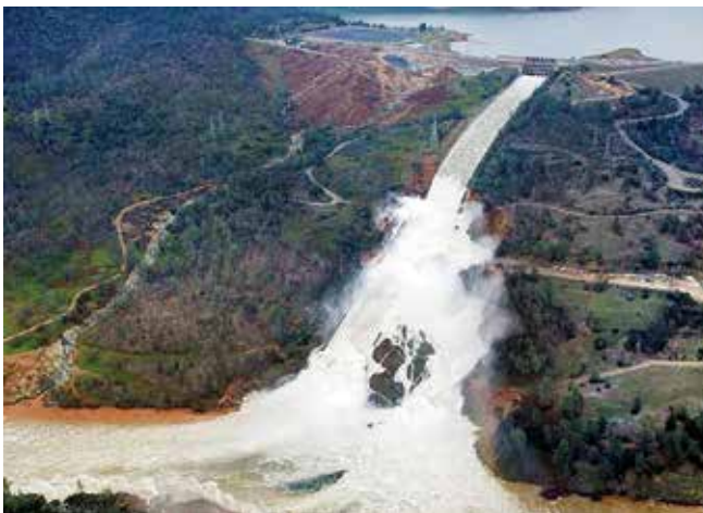
Fig. 1: February 2017 Oroville Dam main spillway is damaged
