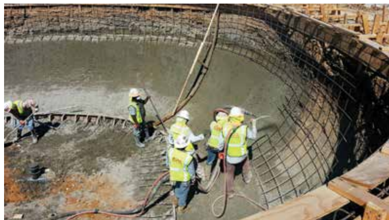
Fig. 3: Proper shotcrete preparation, crew positioning, and concrete placement. An initial layer placed early in the project assures protection of the compacted subgrade from damage due to adverse weather
