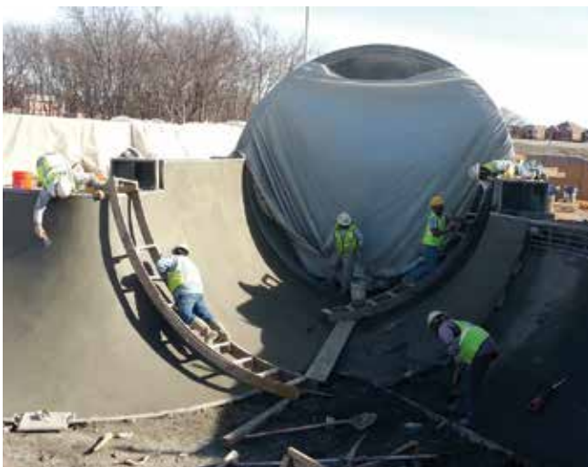
Fig. 5: Second (final) concrete layer with Class A steel-trowelled finish. Over-vertical concrete capsule protected from overspray
