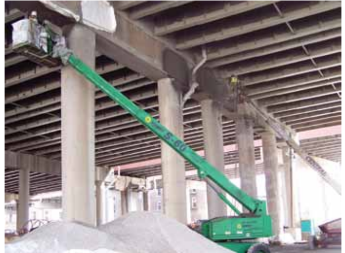
Use of shotcrete over form and pour was chosen for its advantages in "green building"
