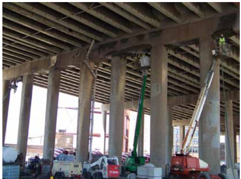
All shotcrete work was done from the ground and pumped upward to the nozzle
