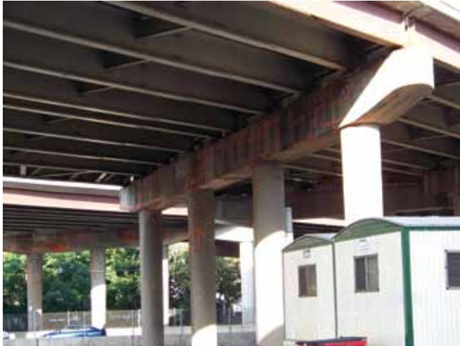
Underneath view of one of the largest and busiest expressways in Chicago, IL
